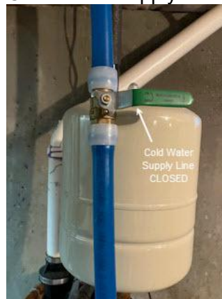
Cold Water Supply Line - Closed
