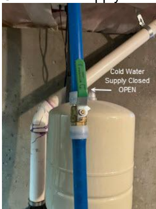
Cold Water Supply Line - Open
