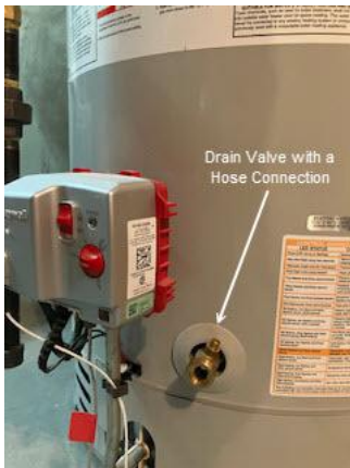
Drain Valve with a Hose Connection
