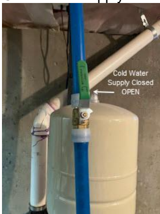
Cold Water Supply Line - Open
