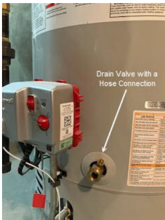
Drain Valve with a Hose Connection
