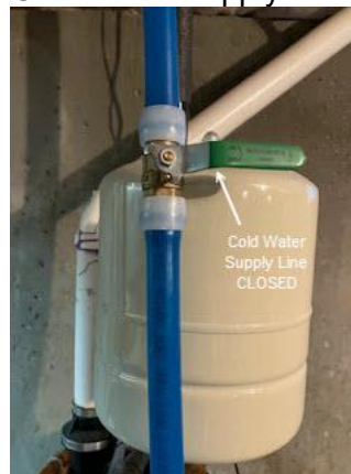
Cold Water Supply Line - Closed
